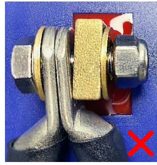
Improper connection for two lugs, top view
